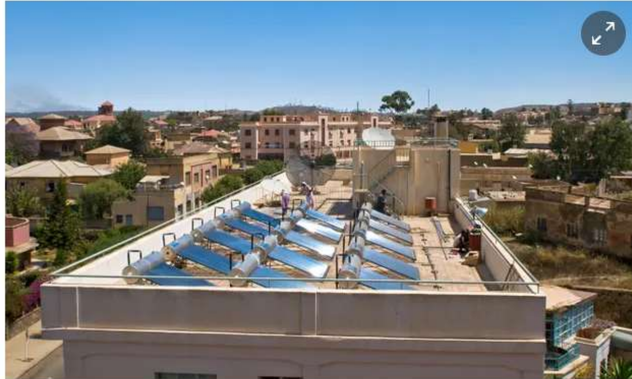
Solar panels in Asmara, Eritrea: renewable power could help cities become carbon zero. Photograph: Sfm Gm World/Alamy
