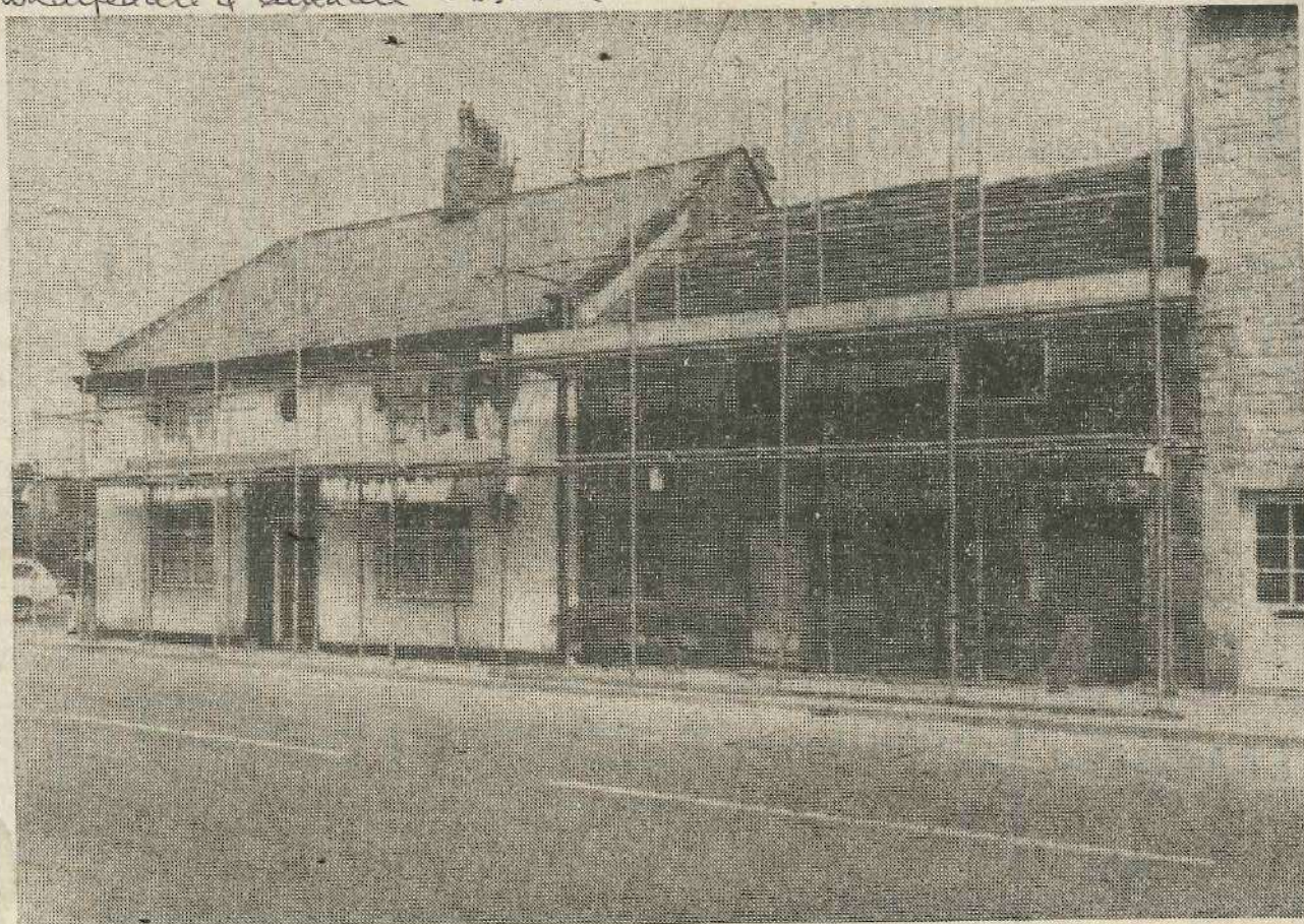
Scaffolding surrounds the Rose and Crown public house in Bondgate, Otley, and the two old cottages into which it will be extended. Engraved in the wall of one of the cottages are the initials
