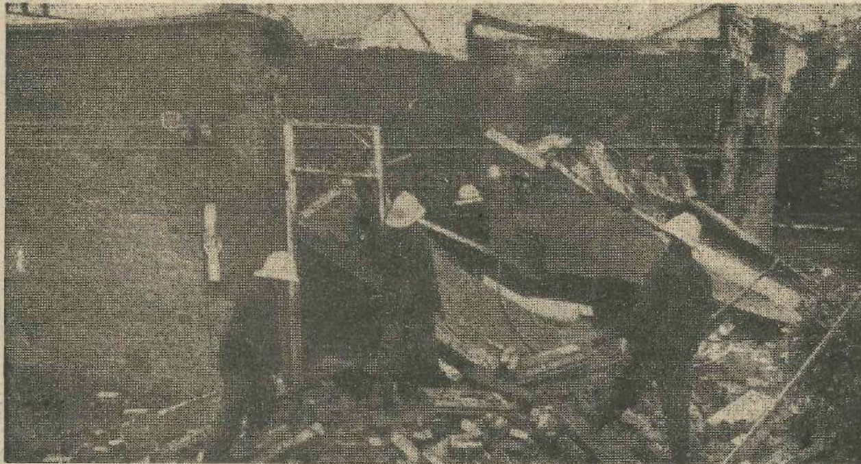
No-one was hurt when an explosion wrecked part of an unmanned electricity sub-station at Easby Drive, Ilkley, causing damage estimated at £15,000. It was believed to have been caused by an overhead cable fault and cut off power supplies to the town for several hours. Picture by Richard Beckwith, Ilkley.
