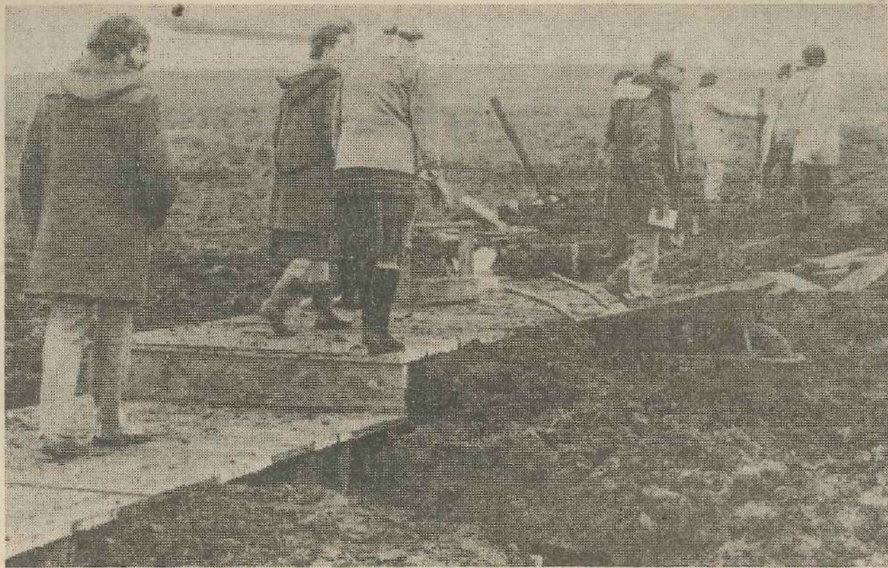
Picture shows work being carried out on the new boardwalk at Dick Hudson's track on top of Ilkley Moor this week.
