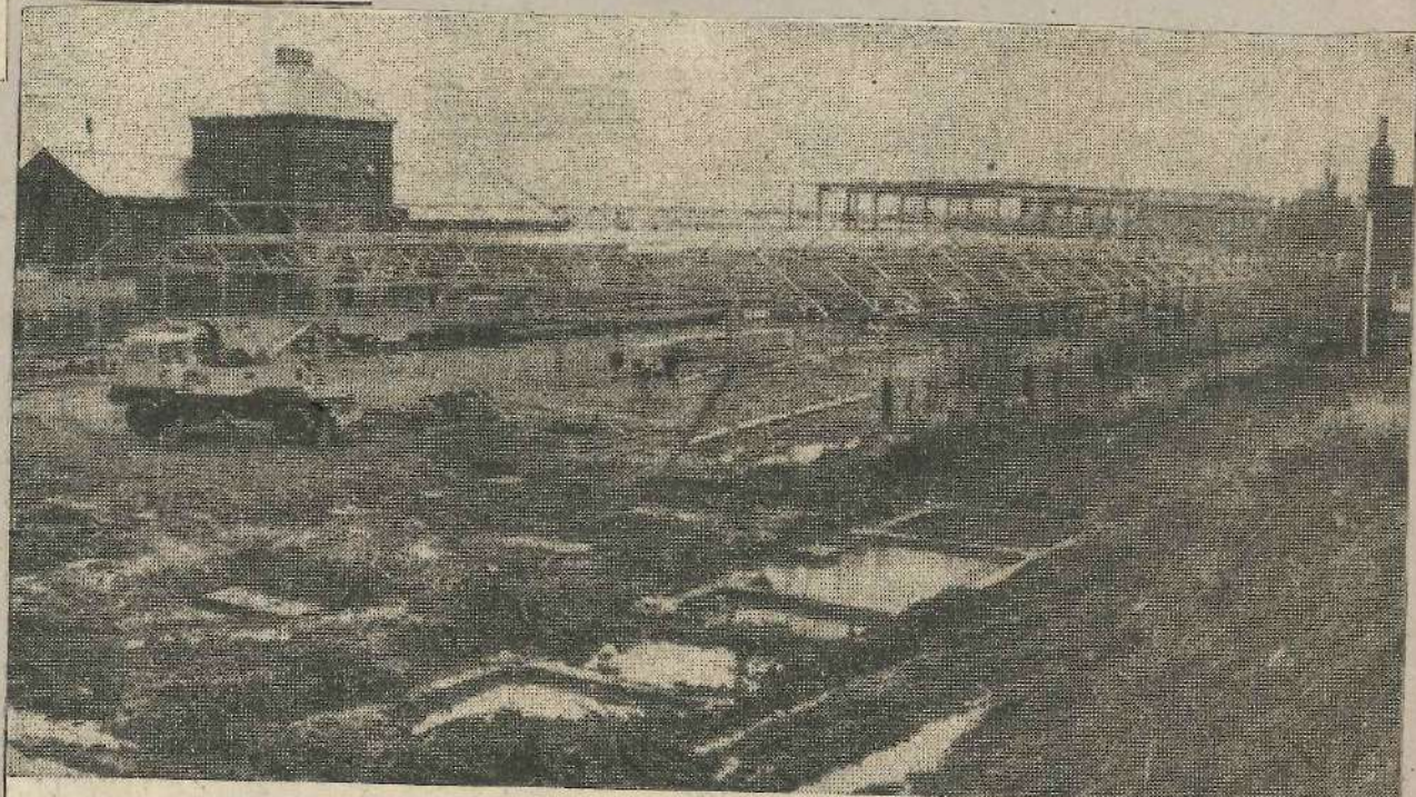
Picture shows work progressing on the office and warehouse block on the site of Hillards' new superstore at Springs Lane, Ilkley.
