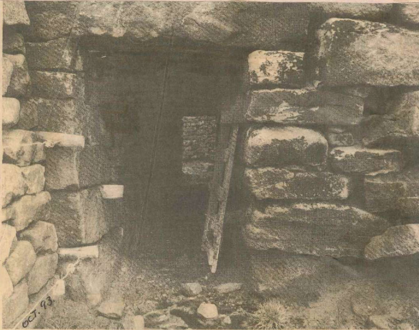
The tunnel under the moor road at Ilkley which farmer Geoffrey Rawson fears could collapse on his sheep because of the number of heavy vehicles using the road.
