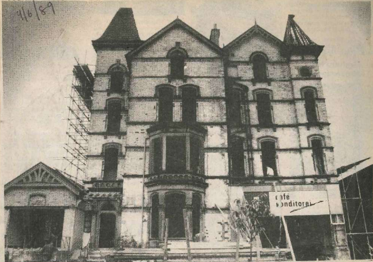
Work on demolishing one of Ilkley's historic town centre landmarks got underway this way this week.
