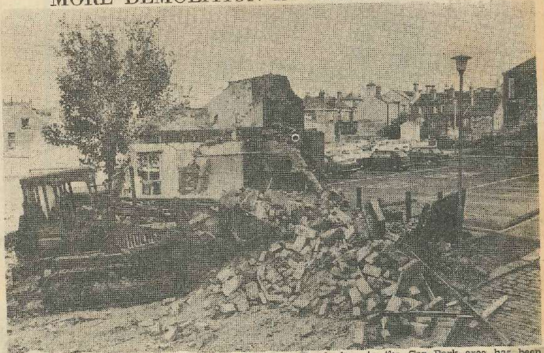
The demolition of other buildings in Back Grove Road close to the Car Park area has been completed recently.
