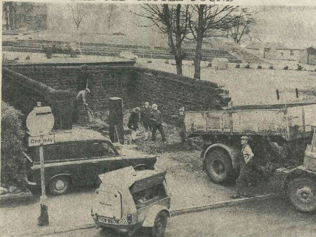
Work in progress at the old cattle pound in Weston Road. The front wall has been removed, the floor of the pound is to be replaced, and the removal of other walls is under consideration.
