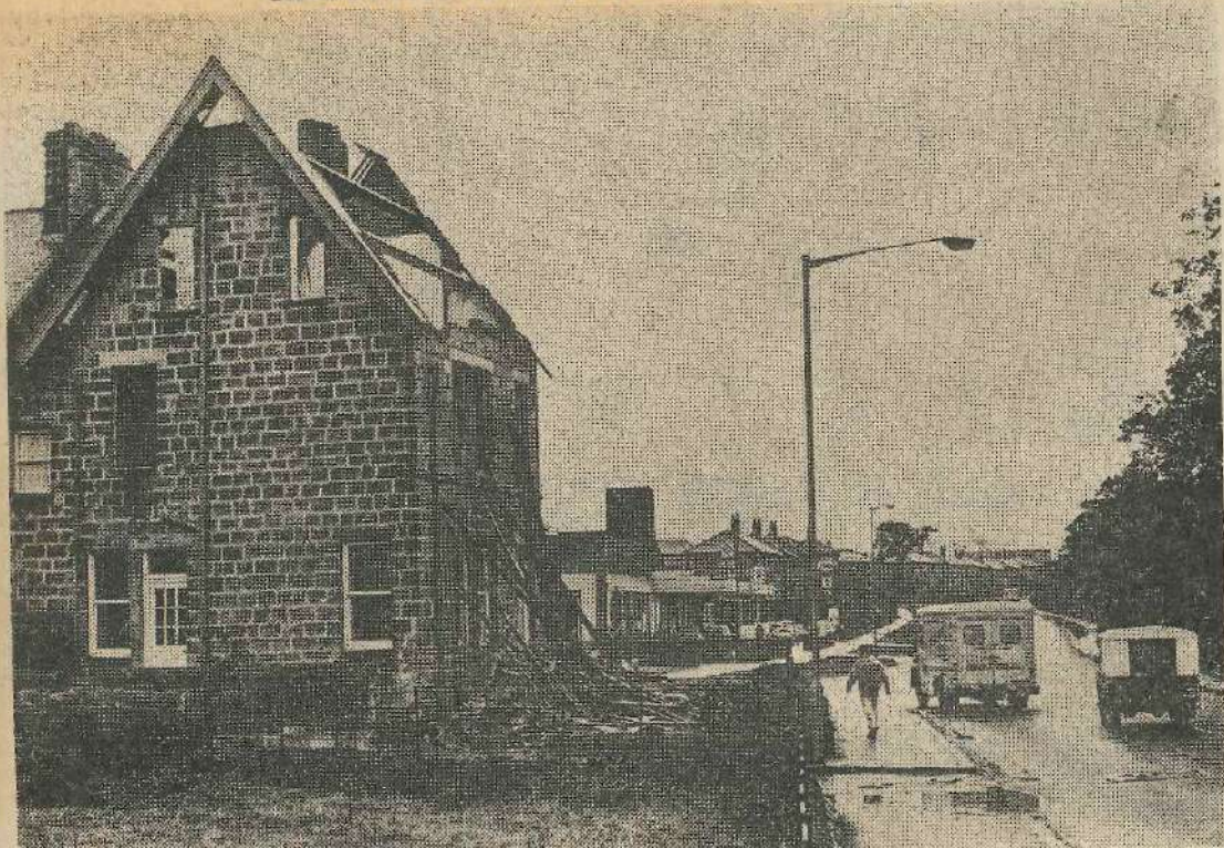
Work began this week on the demolition of the house at the bottom of Wheatley Lane to provide a new slip road for the Ben Rhydding traffic
