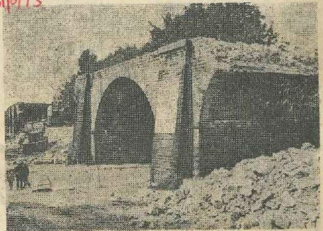
This arch, part of the railway viaduct, over Cunliffe Road was demolished yesterday (Thursday) morning, a group of people assembling to watch it go.
