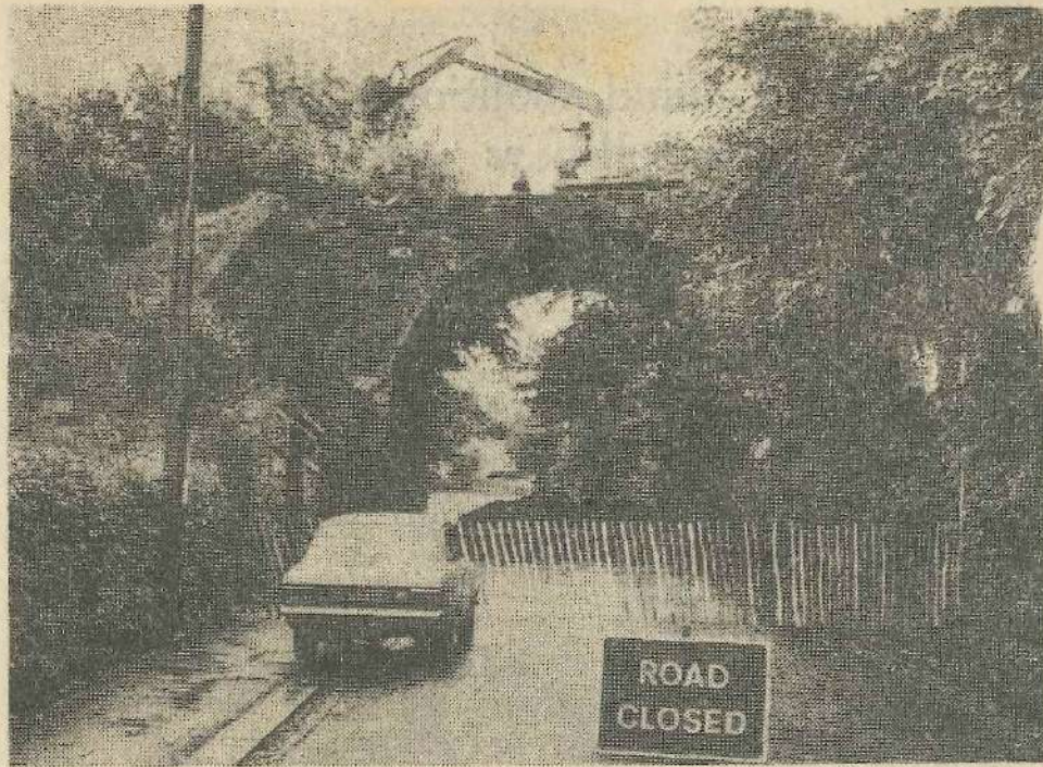
Westville Road was closed to traffic this week as work started on the demolition of the railway bridge. This will be followed shortly by the removal of the embankment and demolition of the viaduct.
