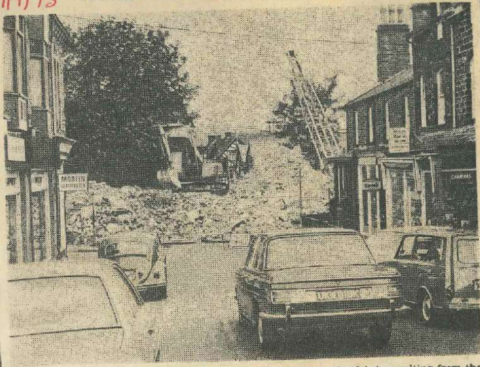
Since last week-end Cunliffe Road has been blocked by the debris resulting from the demolition of the section of the railway viaduct at this point. Traffic has been diverted
