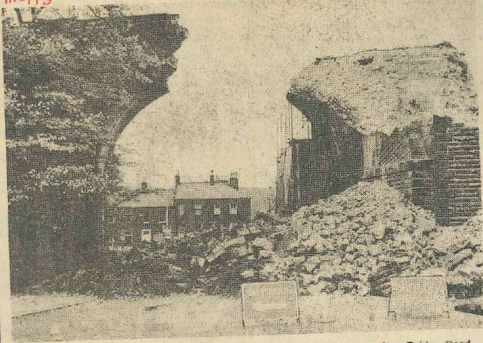
The break through of the arch which carried the railway over Bolton Bridge Road at Ikley. The road is closed to traffic on account of the rubble which falls upon it.
