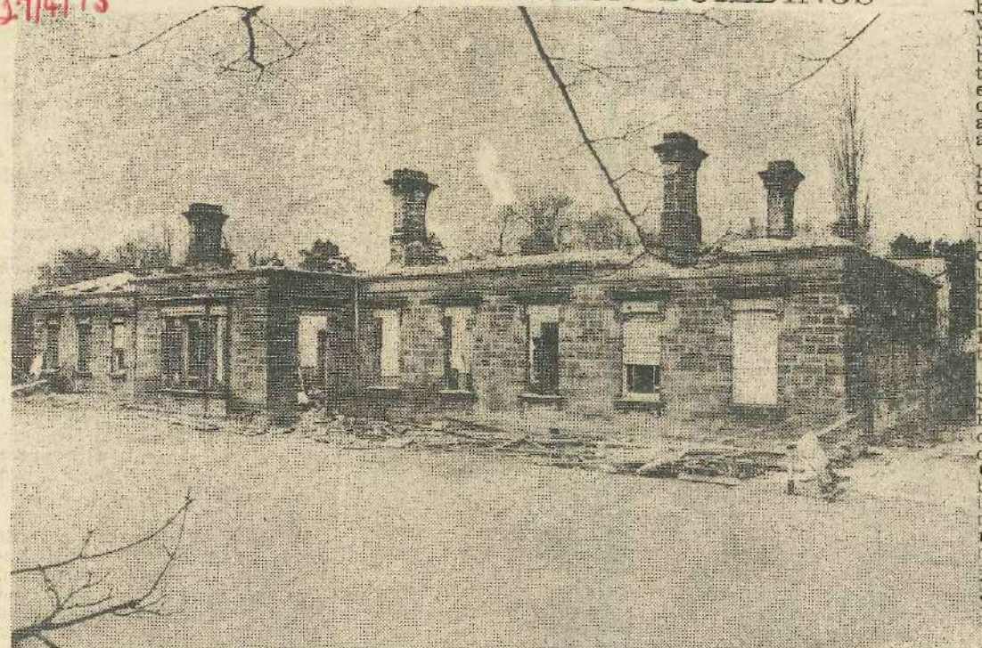
The roof and the interior of the buildings on Burley-in-Wharfedale Station had gone when this picture was taken of demolition work now in progress.
