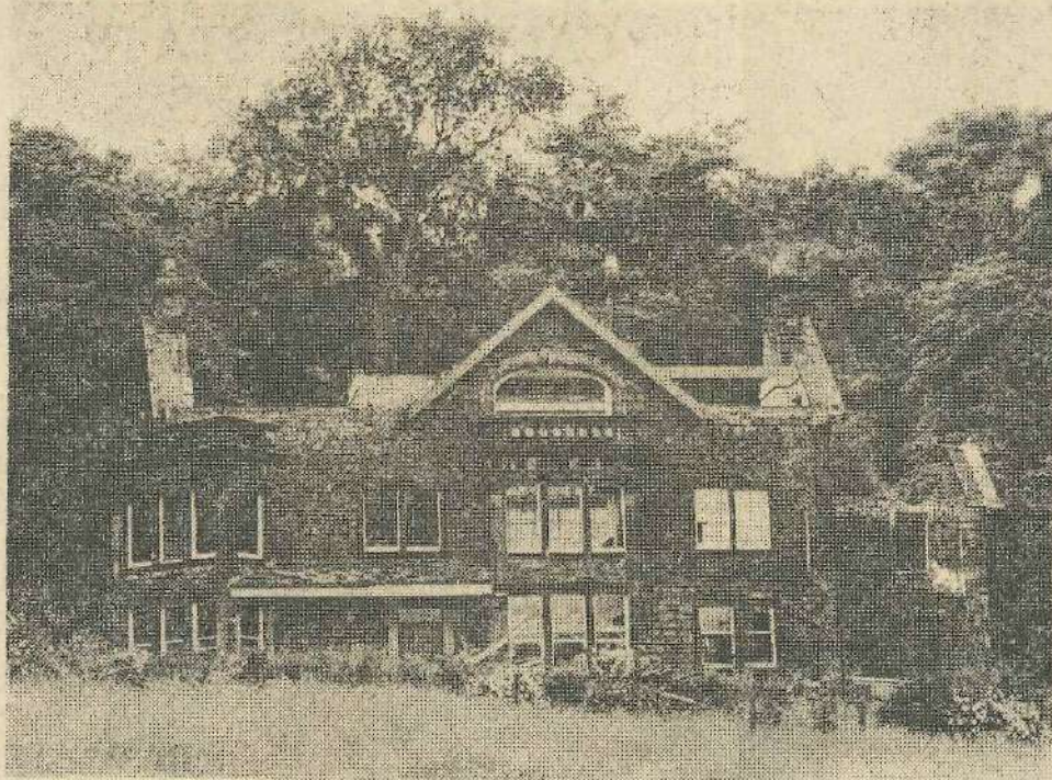
There has been unusual speed in carrying out the decision of the Ilkley Urban Council to demolish Nell Bank, the detached house so ideally sited along Denton Road at Middleton. The slates were off before the end of last week, then the roof timbers removed, and considerable progress has been made since.
