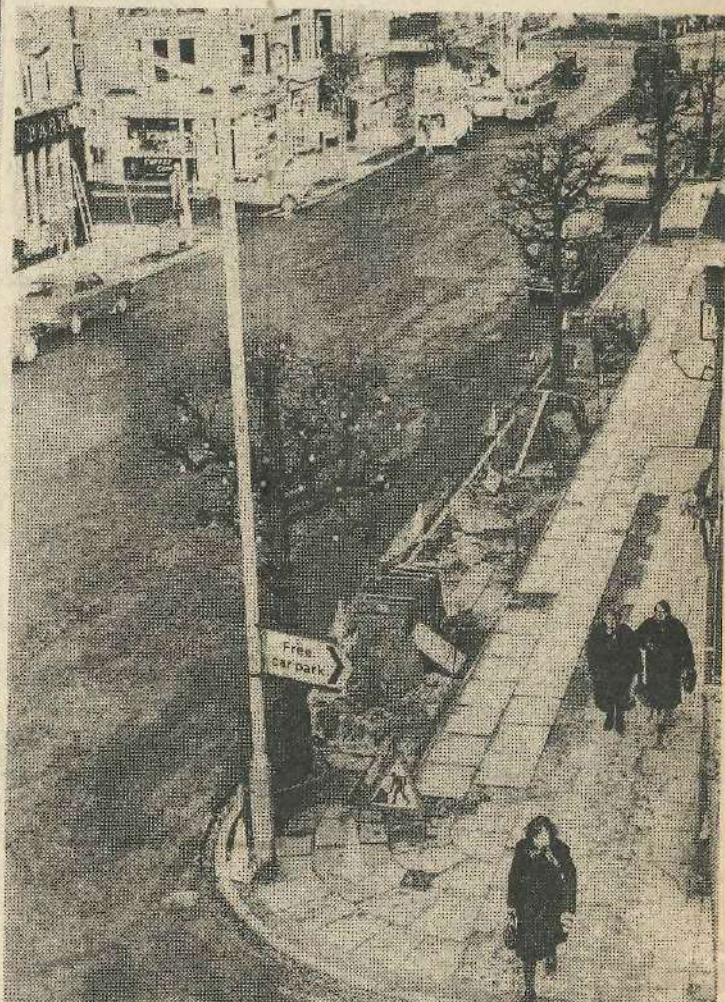
A major scheme of improvements to Brook Street at Ilkley has been in progress for some months. Picture shows the footpath on the east side where work has followed the relaying of the footpath on the west side. The surface of Brook Street itself is also receiving attention this week.
