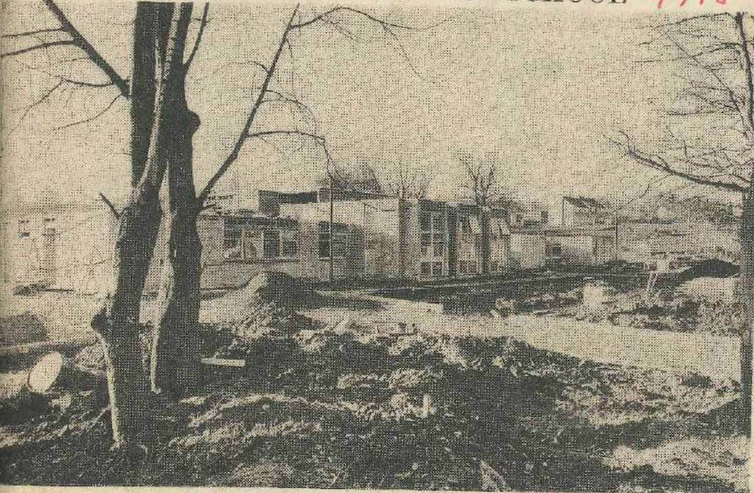
The slow progress made with the erection of the Burley Middle School has been for months the subject of concern for Ilkley Middle and Primary School Governors. At their recent meeting it was reported impossible to indicate any date for the provision of the first phase.
