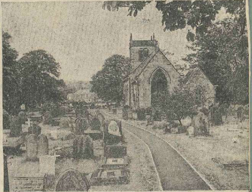
The path in front of St. Peter's Church, Addingham, was relaid with tarmac. For years the path had been made up of gravestones and memorial tablets.
