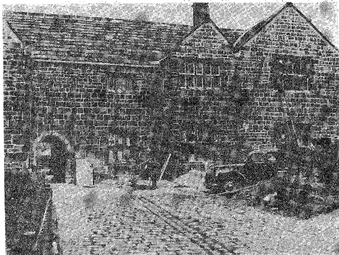
Whilst the work of renovating and converting the Manor House in Castle Yard has been going on, the windows have been systematically broken until hardly a whole pane of glass remains. The job is expected to be completed (with new glass in the windows) next month.
